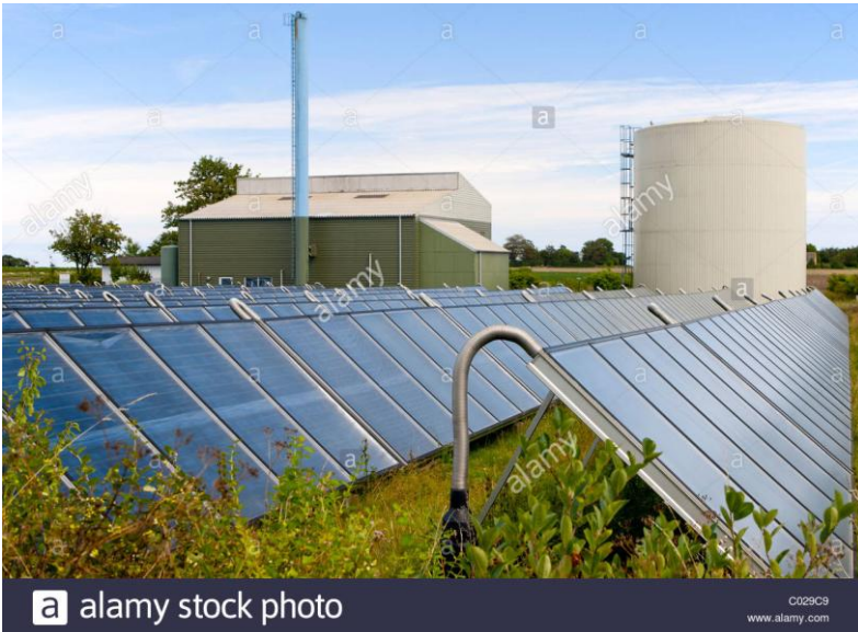
Solar district heating plant, Nordby, Samsoe, Denmark
